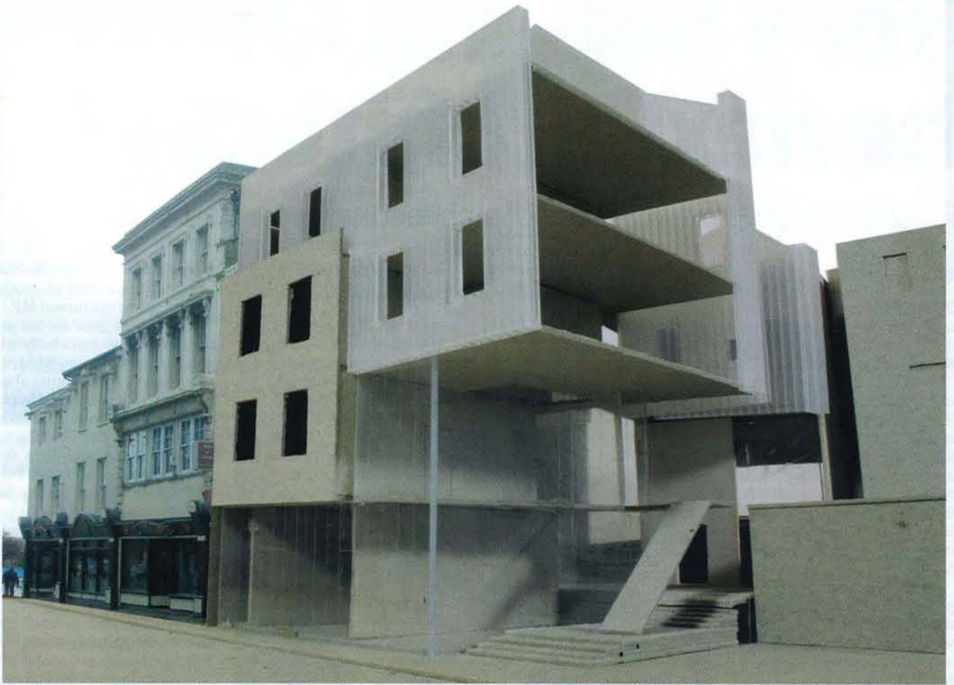
The new Tontine Street building features a polycarbonate panel facade on its top floors.
